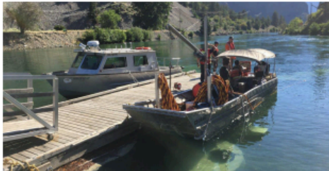
Dive crews prepare for underwater repair work on Seton Lake dock, Lillooet. New dock anchors and chains are visible underwater.
