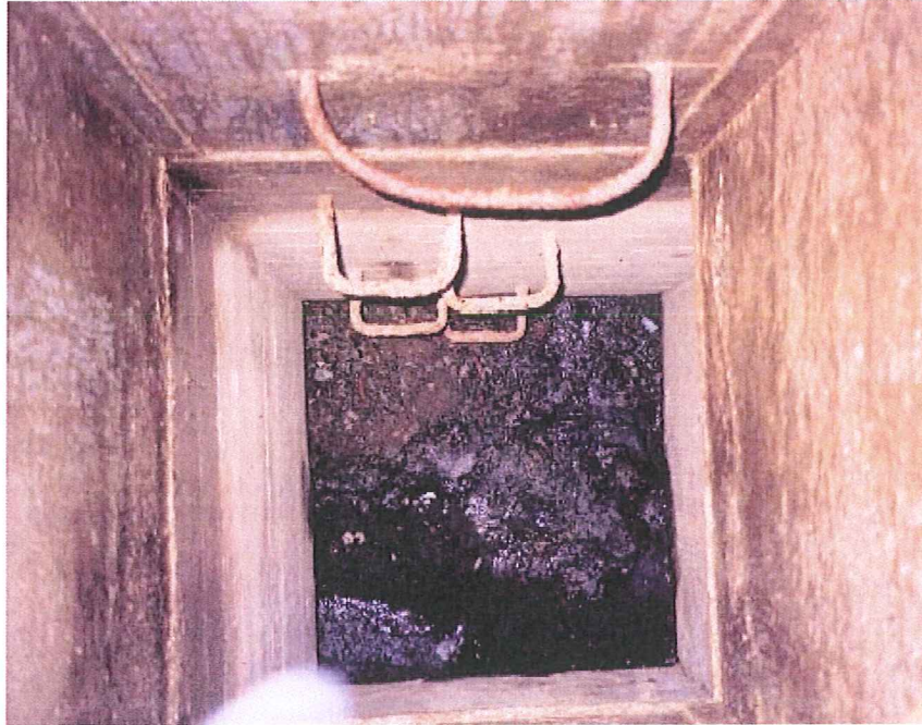
Typical Manhole in Townsite #2 Note Solids Accumulation in Base Area – 2002
