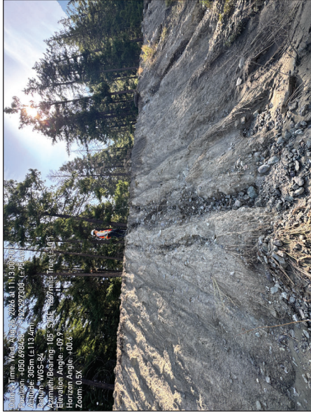
Photo 8. At berm toe looking east at erosional gullies along downhill face of berm at overtopping location.
