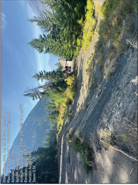
Photo 6. Looking south along downstream berm crest at overtopping location. Occupied residence approx. 30 m downslope of berm.
