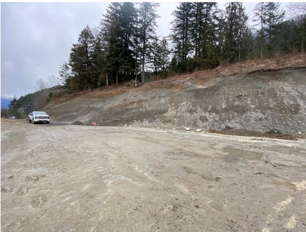
Figure 4 – Photo looking east towards toe of slope where TPs 4-7 were excavated (Area 2). The forested area above the top of bank represents Area 3
