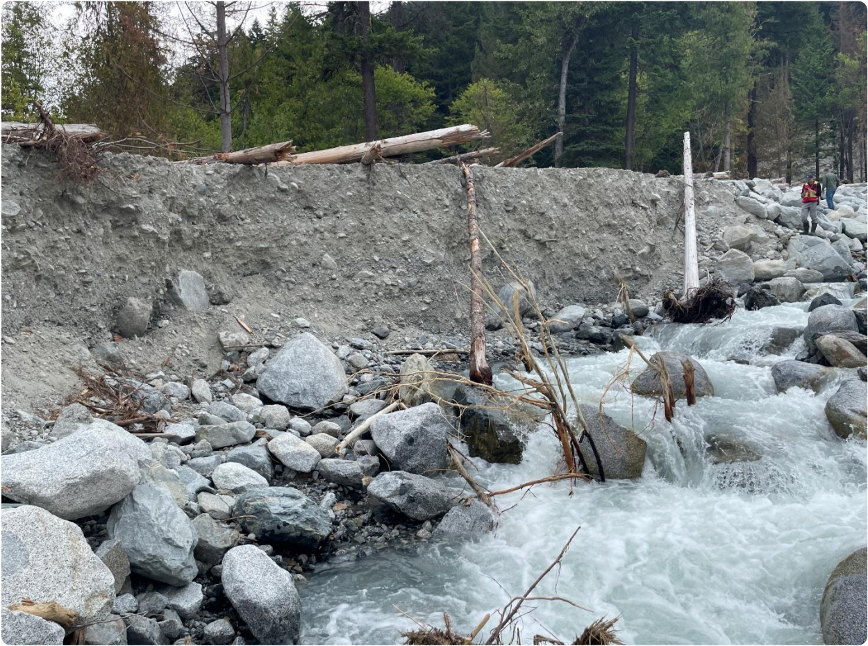
Figure 2-5. Riprap Failure and Embankment Retreat – Looking Upstream (June 8, 2025)
