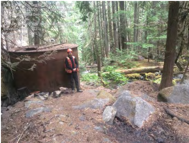
Twin Two Intake, steel tank
