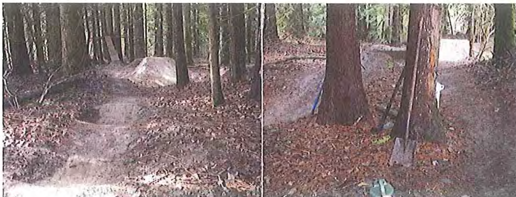
Figure 5: pump track construction within the proposed Riverside Park Photo by Johnny Jones
