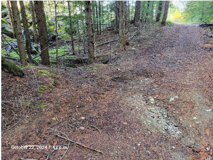
Photo 9. Evidence of erosion observed within the Drainage 2 alignment on the trail. October 22, 2024.
