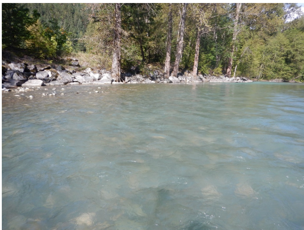
Figure 18 Some armoured and erosion protection on Poleyard Dike and Birkenhead River facing northwest
