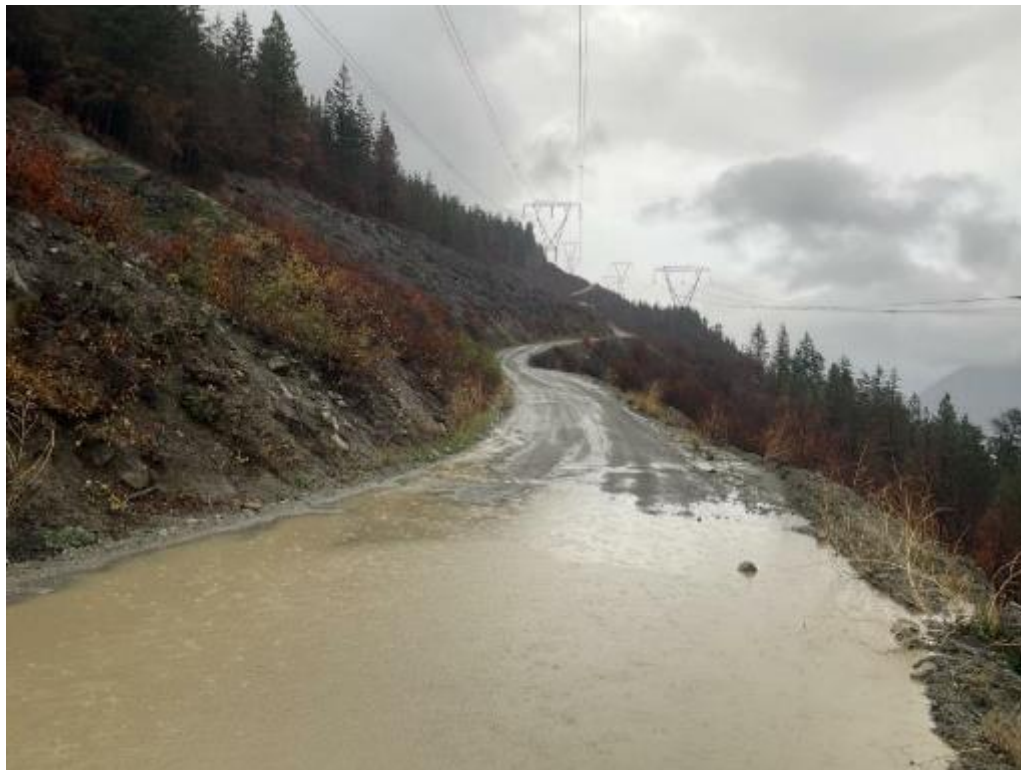
Photo 2 Highline Road flooding near H1 during the atmospheric river event of October 18 th , 2023, looking east.
