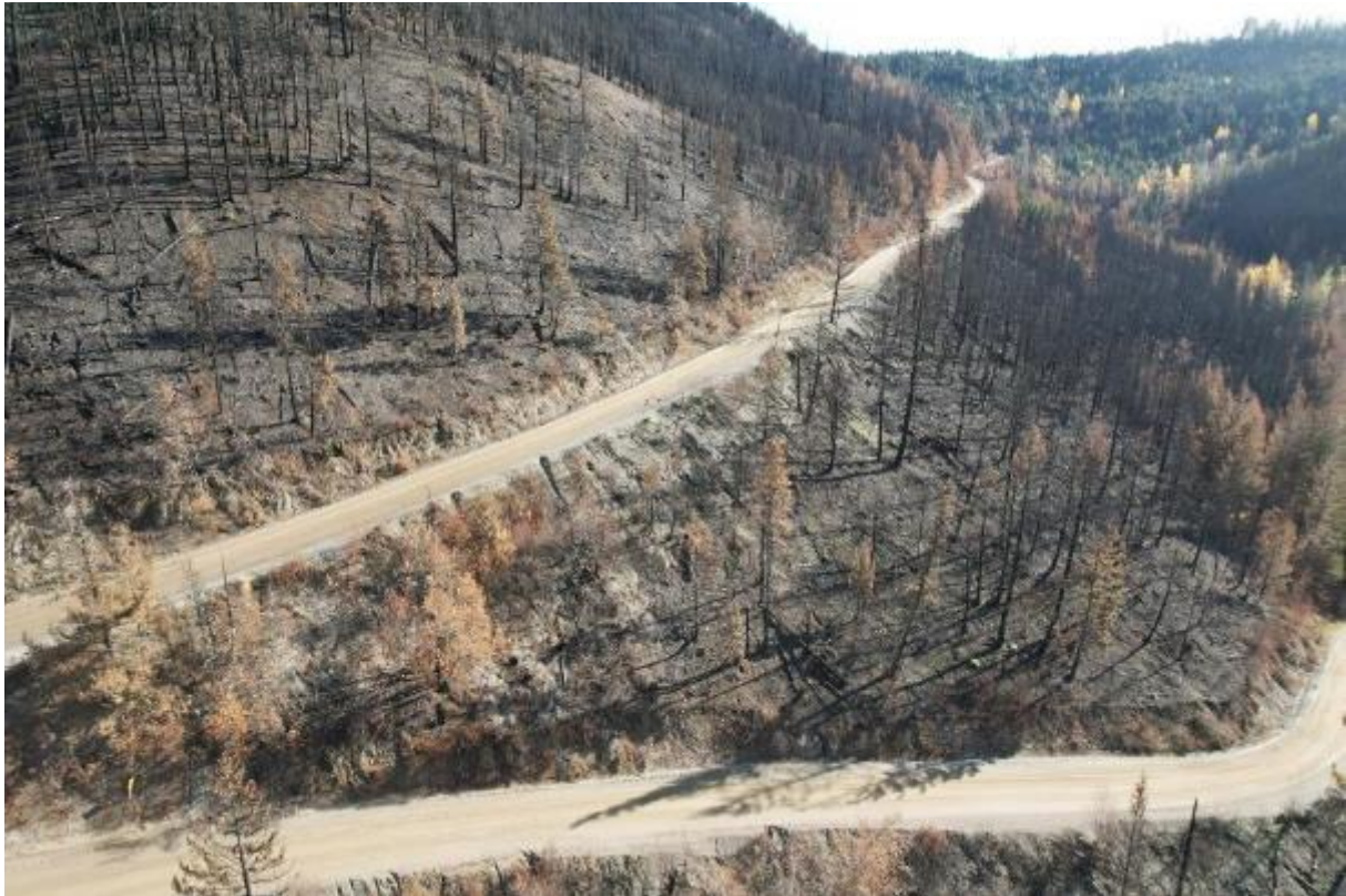
Photo 36 Mission Mountain Road descending towards Carpenter Lake. Note eroded fill in areas of burnt out vegetation in the fill.
