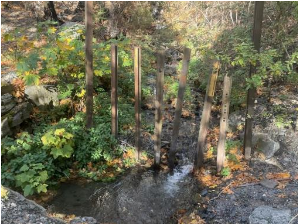
Photo 6 Mitigation structure upstream of culvert inlet at the residential road crossing of H2 at the fan apex.
