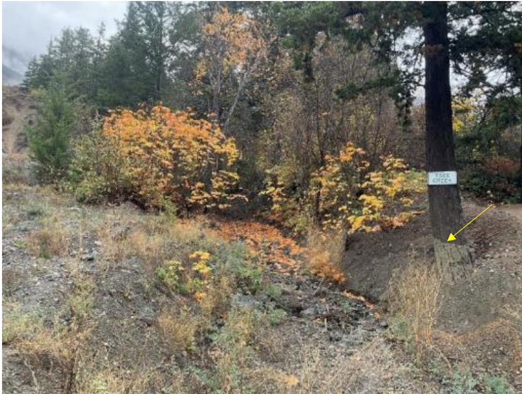
Photo 34 Bedload material and mud splatter on lower Tsee Creek at Shalalth Cutoff Road, looking upstream.
